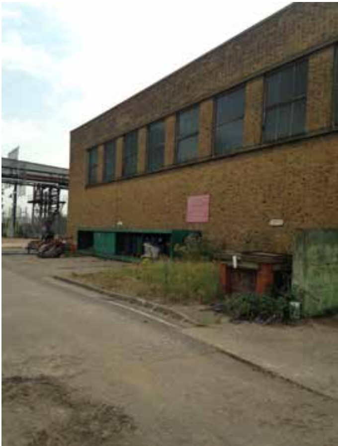
Plate 4: South-east facing photograph of standing Tilbury A structure in south-east of the study site
